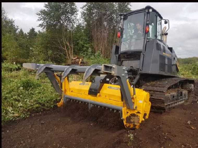
MT-700 with steel tracks and MJHS-2.4 meter crusher clearing dense vegetation. Crusher is equipped with heavy-duty push bar and sizing screen.
